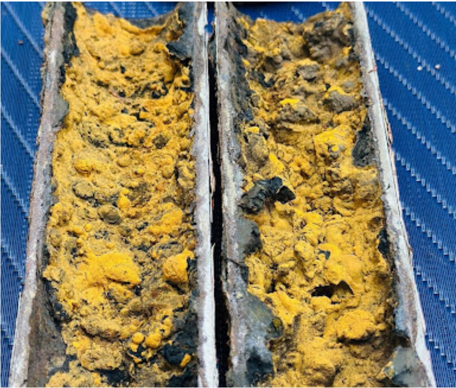
Figure -3 Cross-section of the removed pipeline section illustrating severe internal obstruction caused by corrosion product buildup and localized metal loss beneath deposits.
