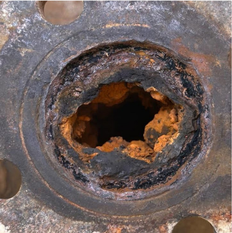
Figure -2 Localized corrosion near a flange connection where flow disturbance and deposit accumulation create conditions favorable for differential aeration corrosion.
