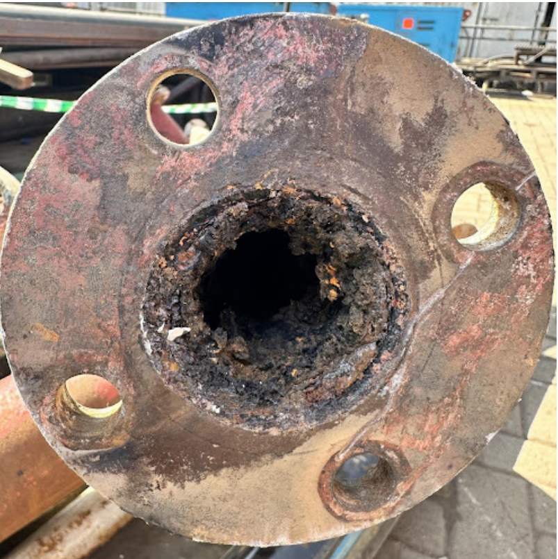
Figure -1 Internal corrosion deposits in the carbon steel pipeline showing extensive tuberculation and significant reduction in the effective internal diameter.
